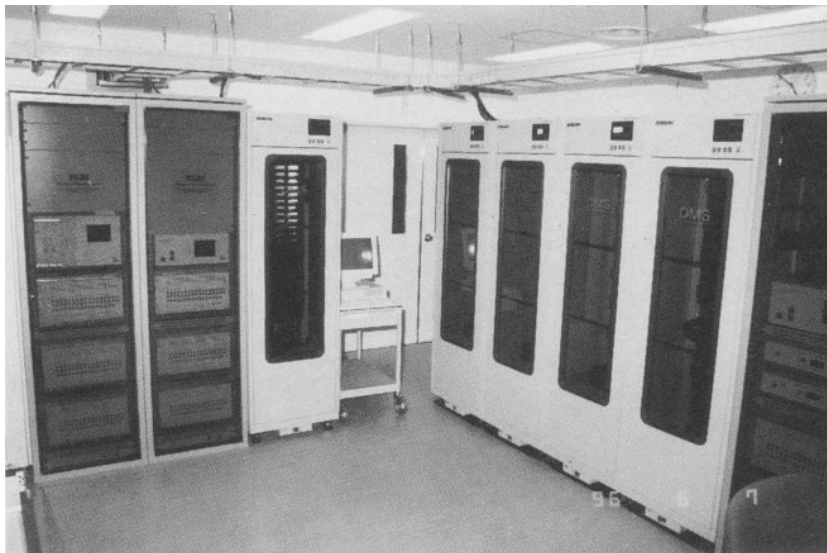
Correlators for the Key Stone Project located in the correlation center at Koganei central station. (Left) Real-time correlators. (Right) Tape-based correlators and automatic tape-exchanger units for each station.(see Page 17)
