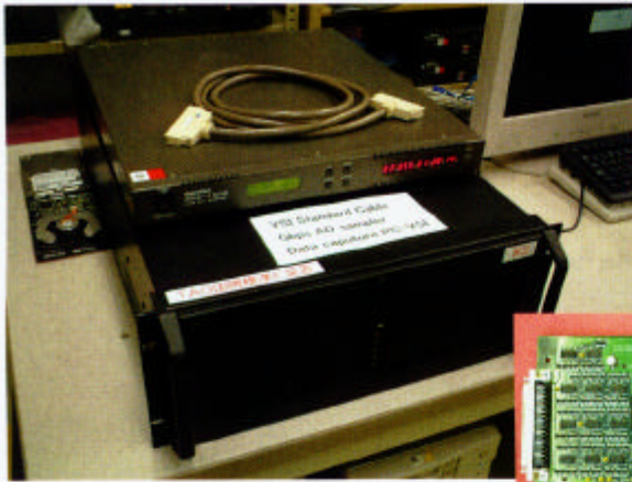
Fig. 1 AD sampler converts telescope receiver output to digital in Gigabits per second. VSI interface board (box) stores Gbps data in PC hard disks. VSI cable connects the instruments.
