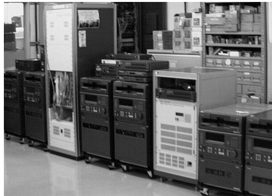
Figure 2. The Giga-bit VLBI system. The system in the left tall rack is GICO-I and that in the right short rack is GICO-II.
