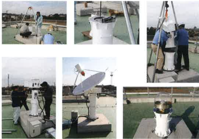
Fig.10 Installation of a first prototype of the compact VLBI system on the top of the 34 m antenna building on December 9, 2008 at Kashima
