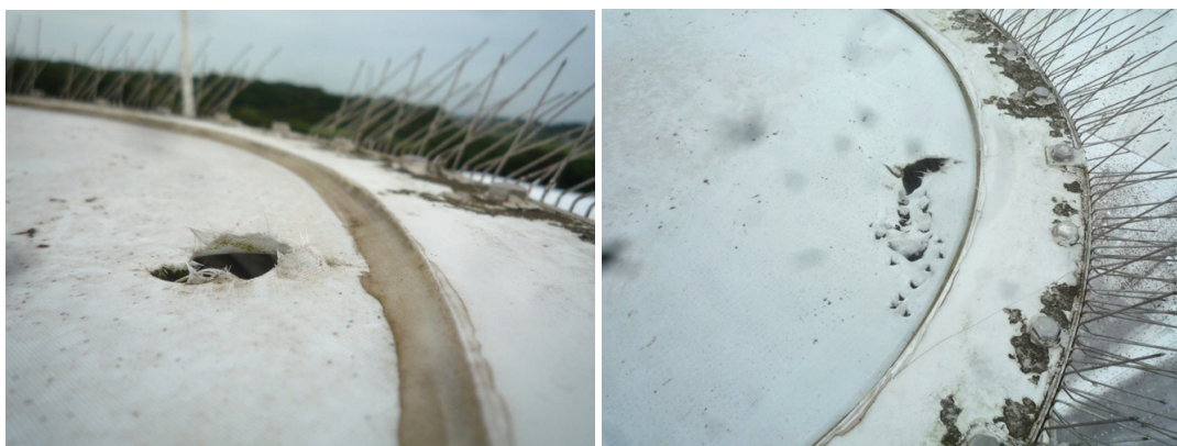
Fig. 3 A hole was found on the feedome sheet of Kashima 11-m antenna in July (left). The hole was closed by tentative repair. However, additional holes were found in August (right).
